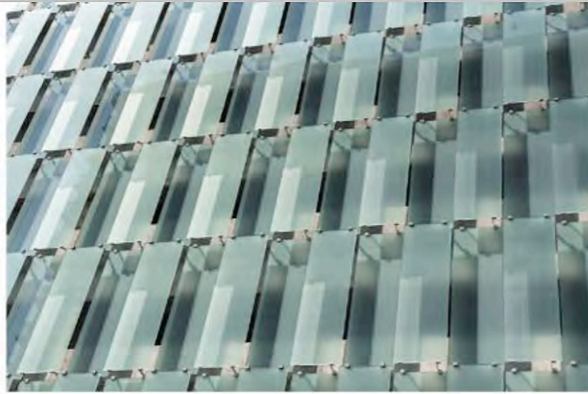
The open-ventilated north and south elevations comprise white laminated glass panels in two levels of opacity.
